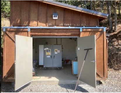
Left: Pine Grove Reservoir Right: Pine Crest Pump Station
